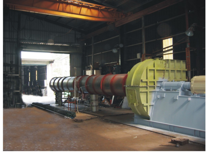
ON-FACTORY PERFORMANCE TEST OF 250 HP ID FAN
